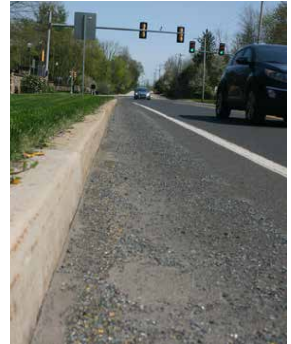
Regular sweeping of a roadway's edge ensures that shoulders and bicycle lanes remain usable.
